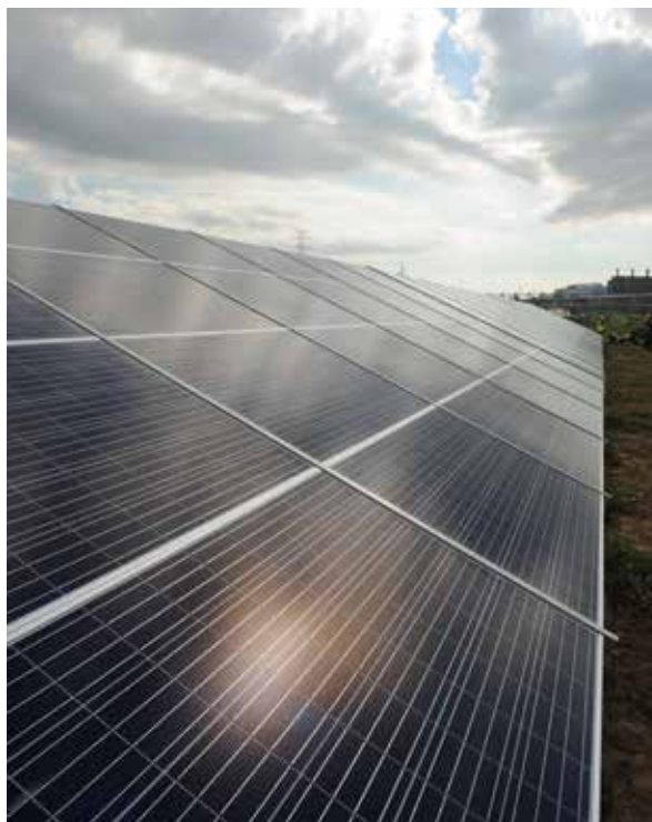
Photovoltaic plant on the site « SAFEA » in La Louviere
